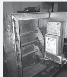
Problem: Failed motor
